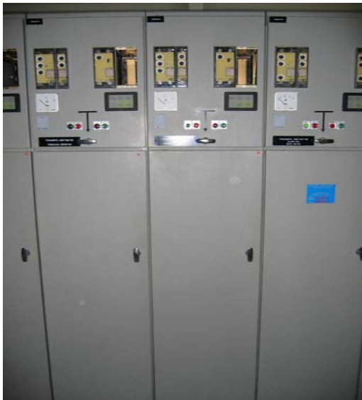
Existing 18 kV cubicle
