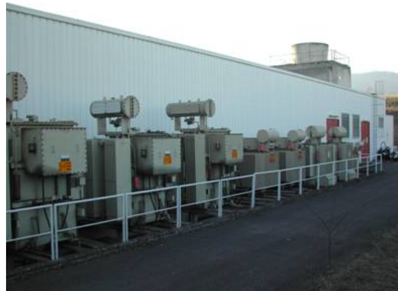
Existing transformer pit
