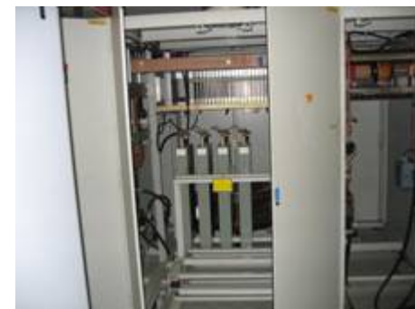
Passive filter capacitors
