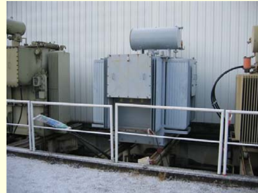
AC transfo outside build.193
