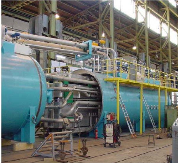
Large Scale Helium Refrigerator by Linde: 18 kW for CERN - LHC
