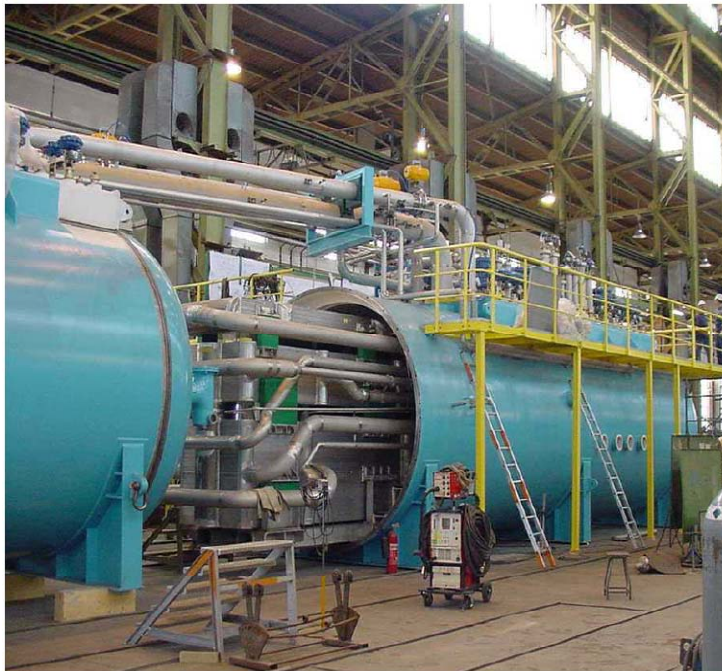
Large Scale Helium Refrigerator by Linde: 18 kW for CERN - LHC
