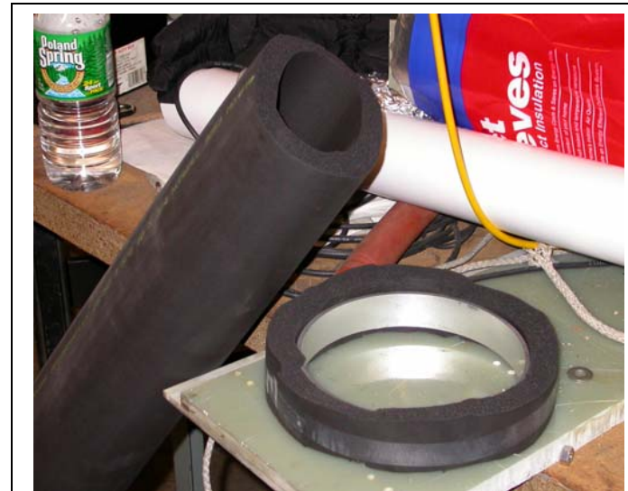
Armaflex insulation on a ring section of the vent pipe Two segments of smaller diameter pipe insulation is used for the 6 inch vent
