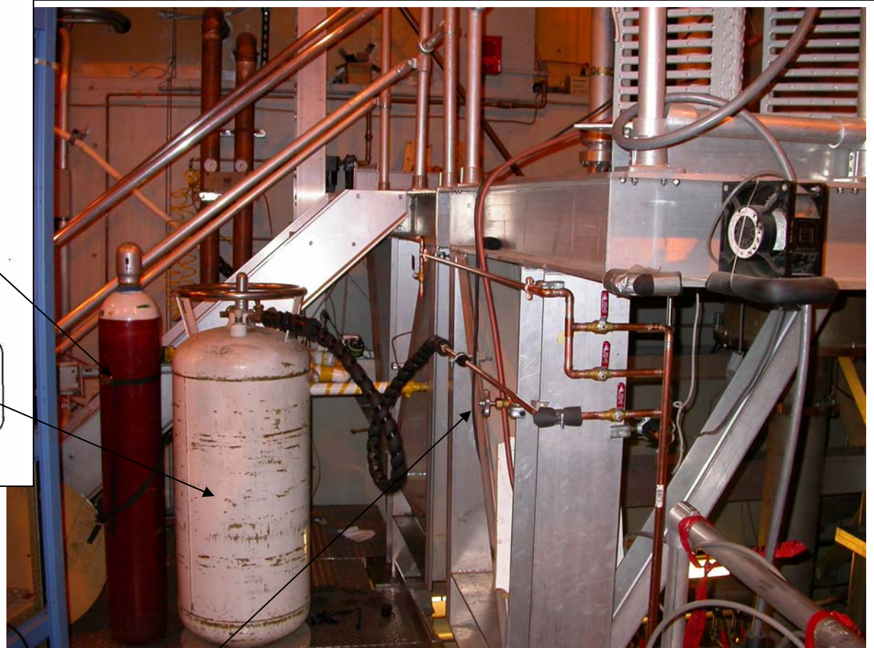
Main LN2 Control Valve. (Long Stem Cryo Valve)
