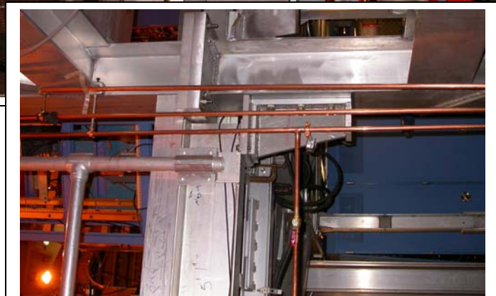
Gas Lines and N2 Gas Volume Measuring Line
