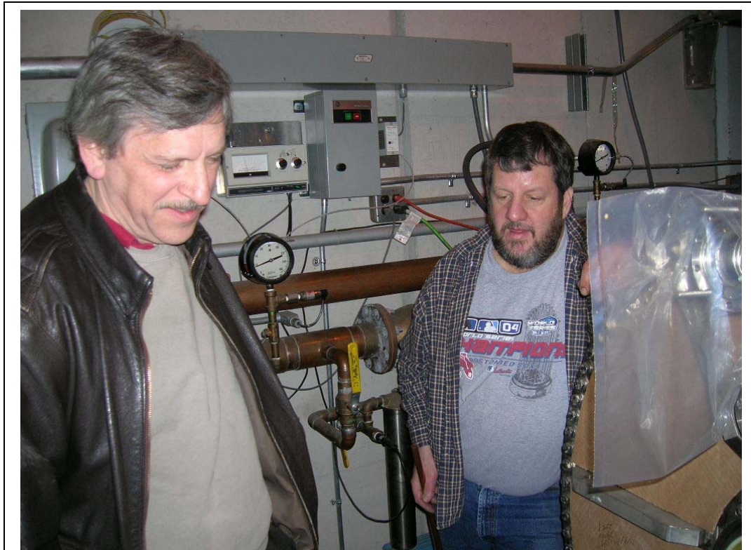
Peter Titus and Dave Tracey inspecting terminal ends of the MERIT Pulsed Magnet –In PTF Facility at MIT-PSFC
