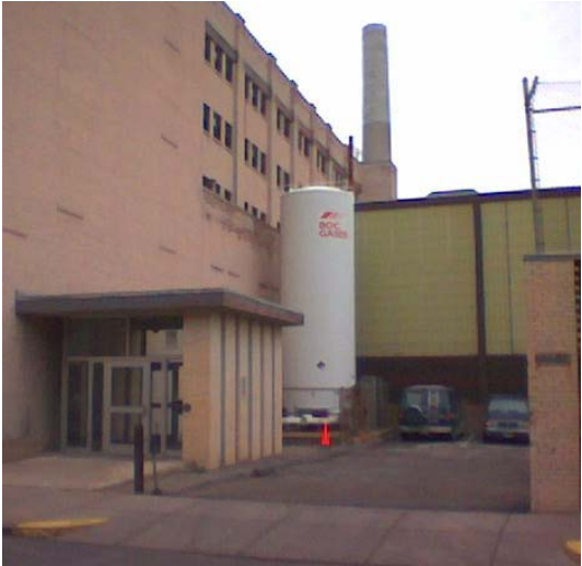
Magnet Lab's LN2 Supply Tank
