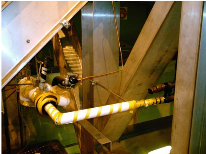
LN2 Supply. –This was disconnected by LDX and will be re-connected.
