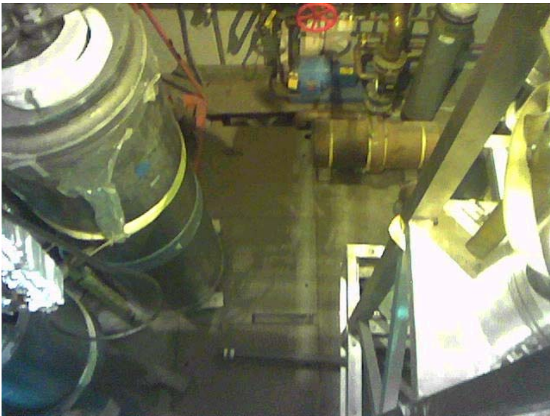
View of the test area floor. The dewars at left and HCX components at right need to be removed
