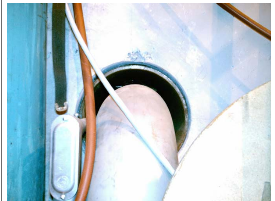
Annular space around water line proposed for use with the gaseous N 2 vent.
