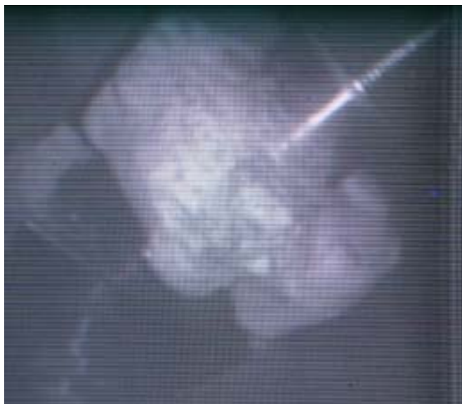
EVAC NW25 chain clamp at lower beam left port, covered with corrosion from water leak in Al seal.
