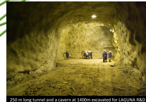
250 m long tunnel and a cavern at 1400m excavated for LAGUNA R&D
