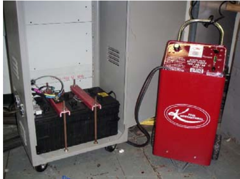
Battery/Charger 12V 1400A
